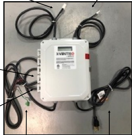
Meridian Control Panel
